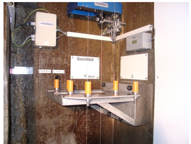
Console for plumb wire measuring system
